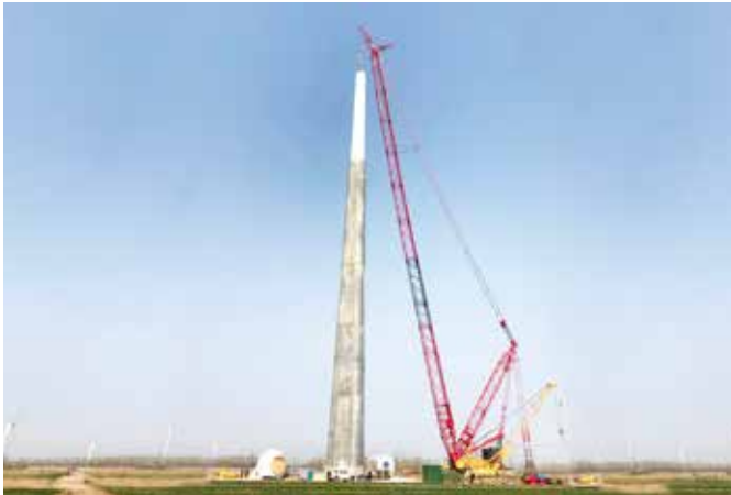
BASF grouting solutions enabled the construction of a 120m concrete-steel hybrid tower, a milestone in the history of wind power.
