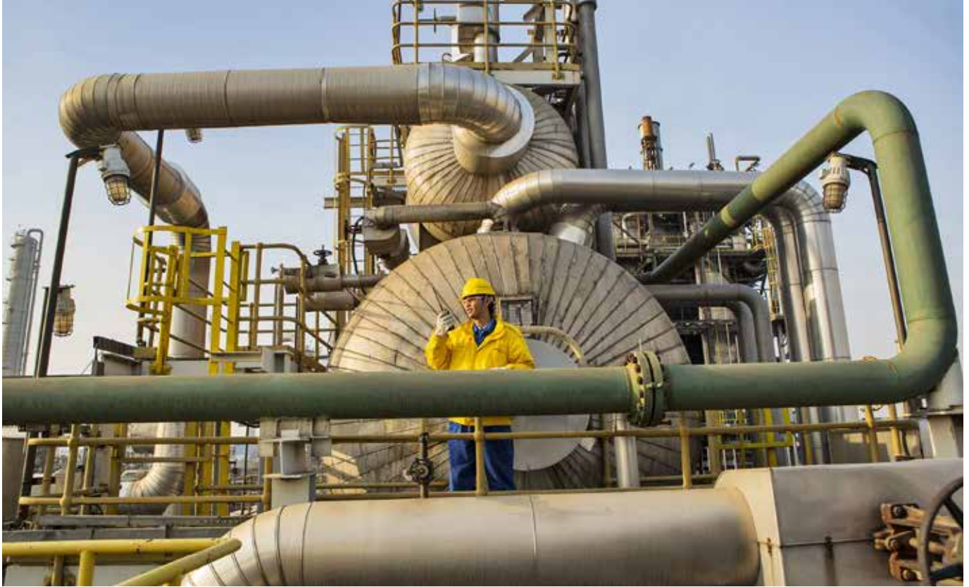
An operator conducts a routine inspection at BASF Nanjing Verbund site. Production plants are linked together via a network of pipelines. This saves costs and increases energy efficiency.
