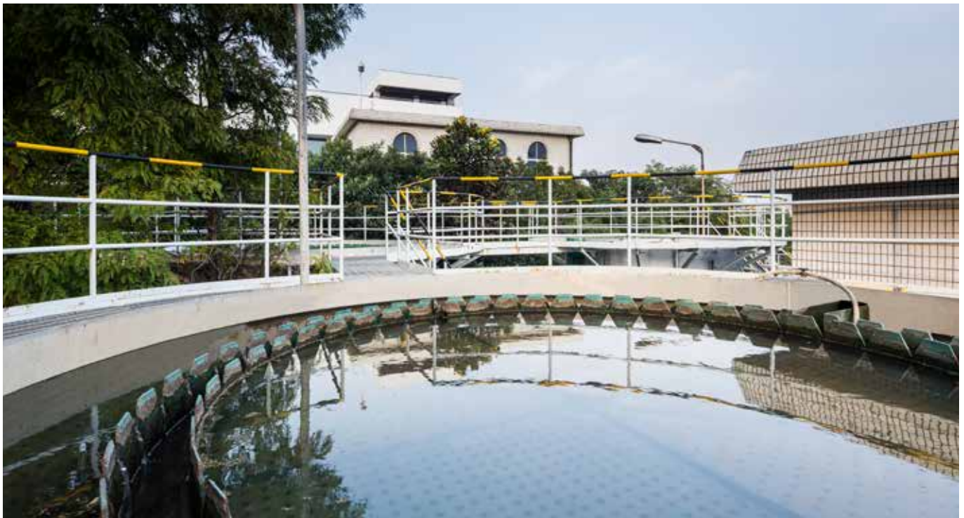
Wastewater treatment station at BASF Shanghai Pudong Innovation Park
