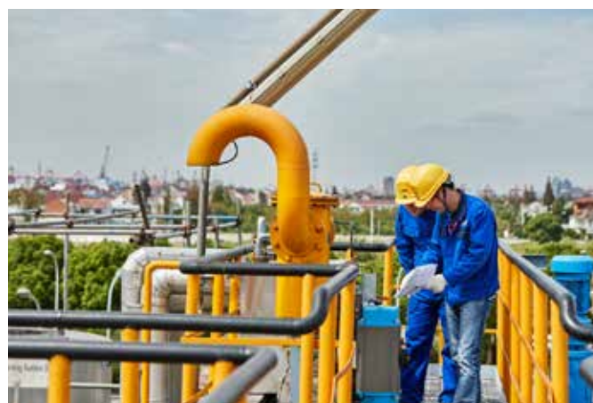
Two operators inspect the off-gas emission point (the orange pipe). The gas has been treated within the facility before being released at this point.
